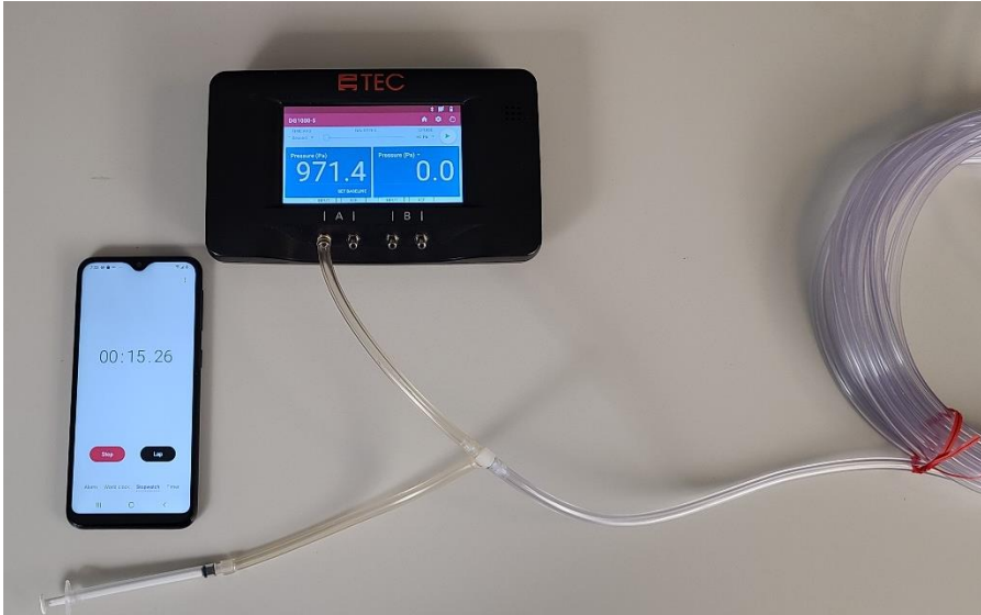
This sensor measures 971 Pa after 15 seconds. It passes the leak test.
